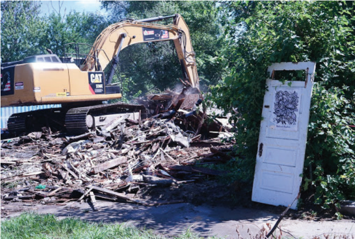
Moments after the house was demolished, a single door with a piece of art preserved.
