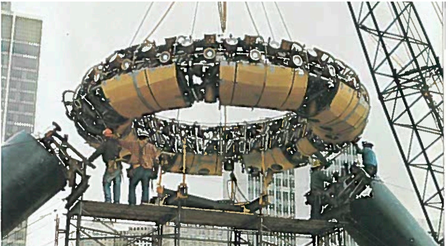
Horace E. Dodge and Son Memorial Fountain being installed. 1972-1978 Detroit Civic Center Plaza
